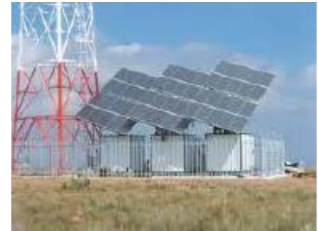
Solar powered cell tower
