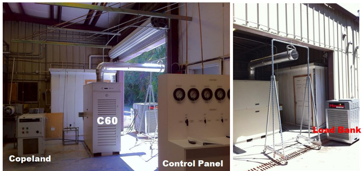
Figure 7: Micro-turbine test system
