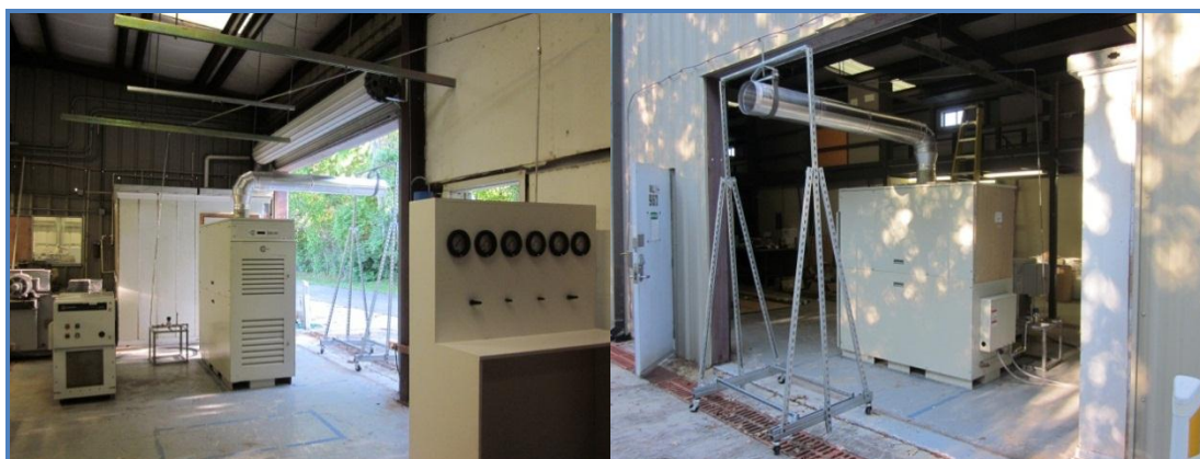
Fig. 1. Micro-turbine test system photograph
