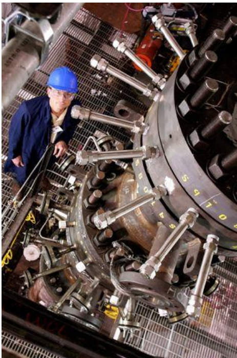
PWR's compact gasifier located at their pilot plant in Des Plaines, IL.
