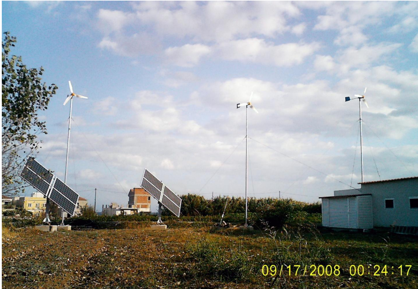
1 kw model in operation (hybrid system with solar panels)
