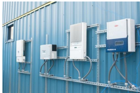
Figure 7: PV Inverter Testing
