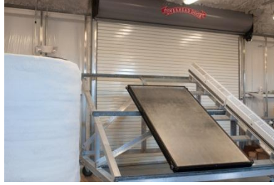
Figure 5: Solar Thermal Testing Lab
