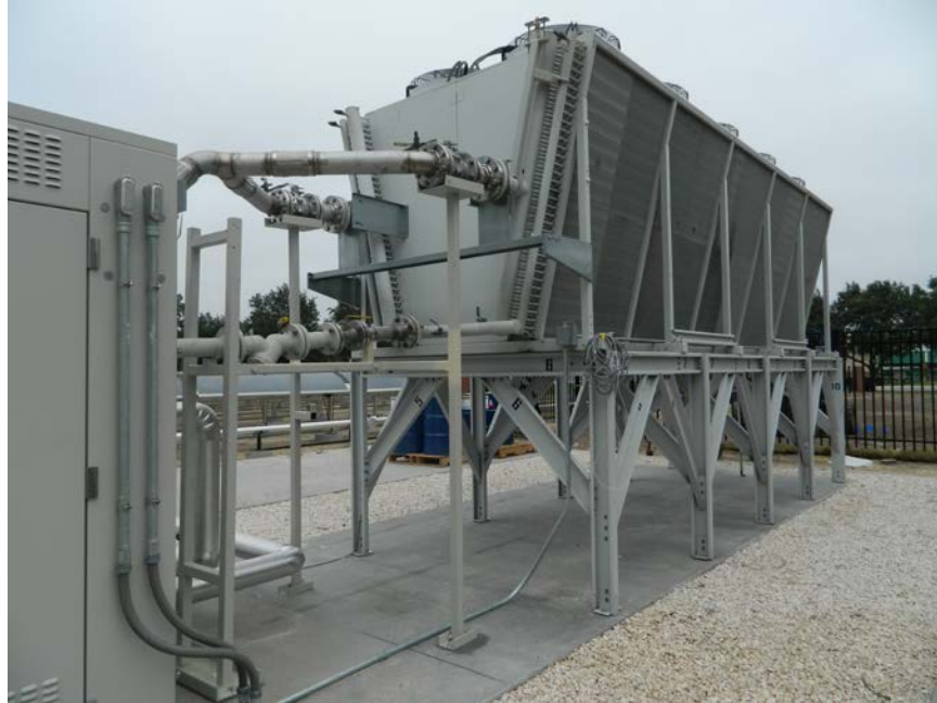
Fig. 12 Electratherm power generator with air-cooled condenser.
