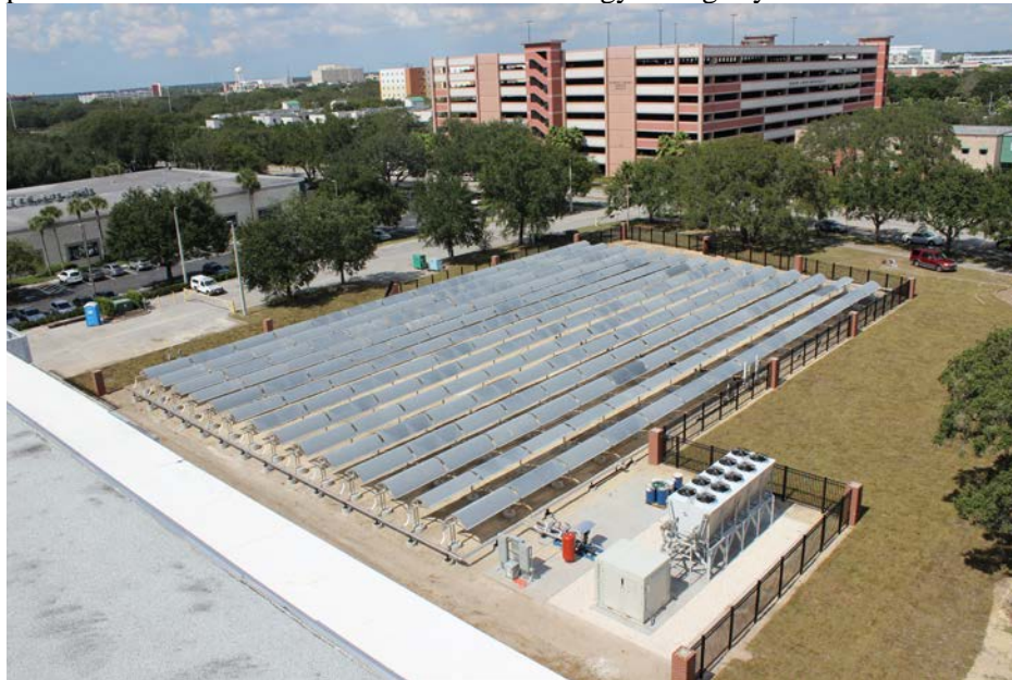
Figure 1. Solar Field and power block for the 50 kW e power generation system
