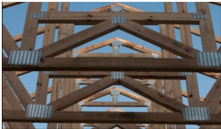
Figure 6. (right) Rafter design allows for a walkway above insulation level for easier attic walking for experiment changes.
