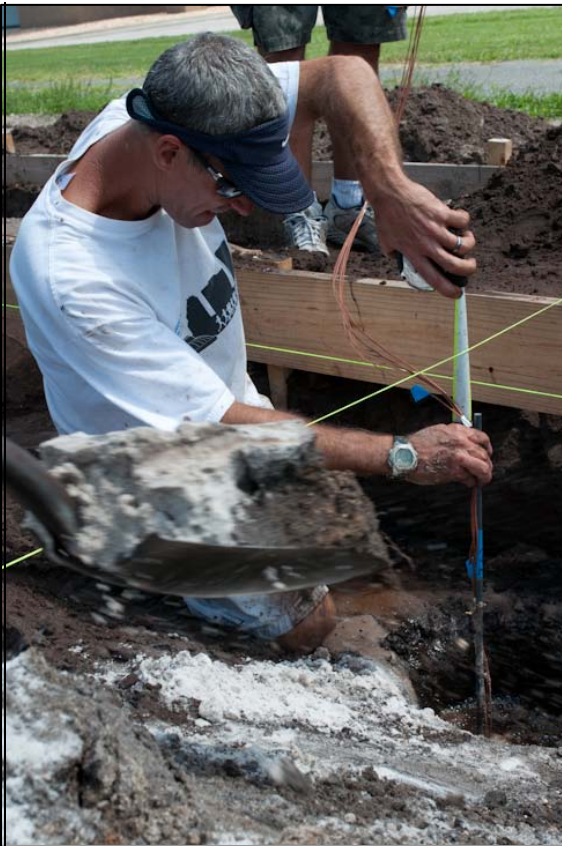
Figure 4. FSEC's John Sherwin measures for exact depth placement; yellow strings mark top of slab.
