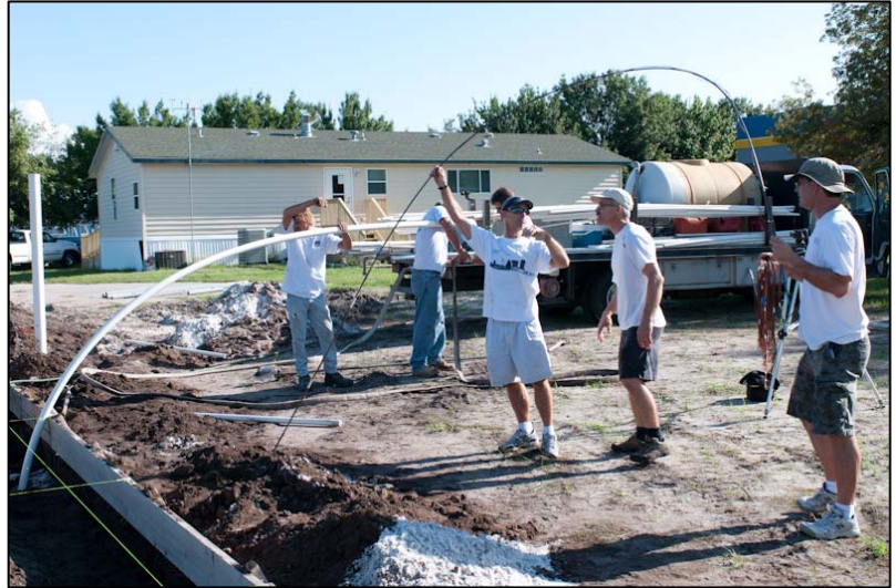
Figure 3. (above) PVC rod with thermocouples tied to it is lowered into hole.
