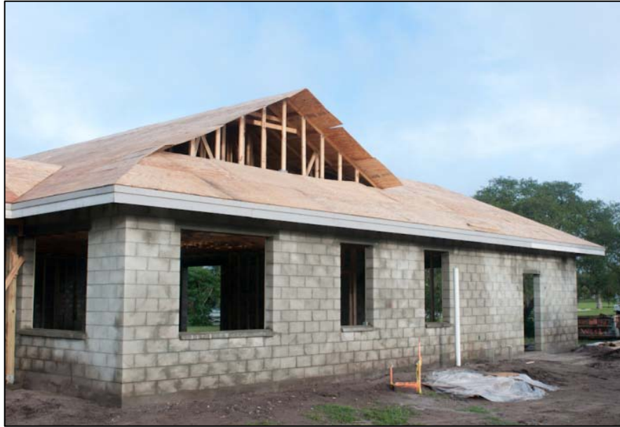
Figure 7. September 30 photos shows plywood sheathing near completion. Dutch hip roof design allows for overhang on all four sides while providing an attic ridge area as well.
