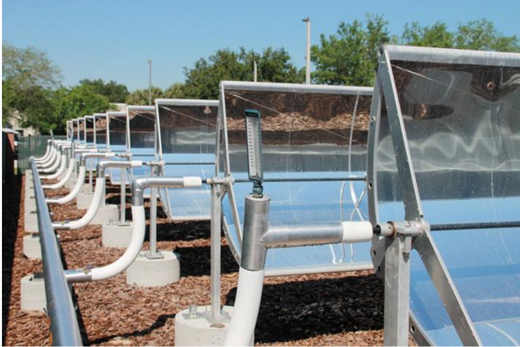
Fig. 3 Solar collectors showing the header connections
