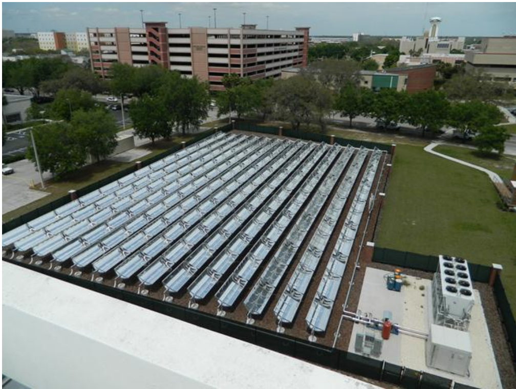
Fig. 1. Solar Field for 50 kW e power generation
