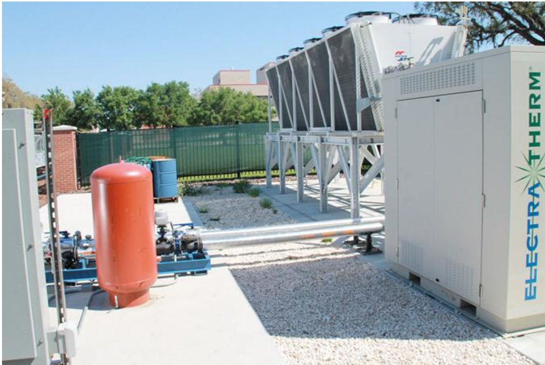
Fig. 2 Power block with air-cooled condenser
