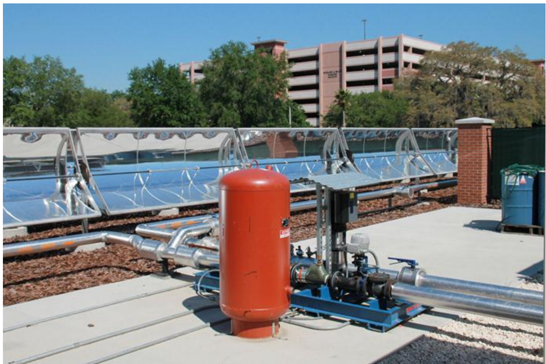
Fig. 6 Pump, piping and expansion tank for heat transfer fluid flow to and from the collector field
