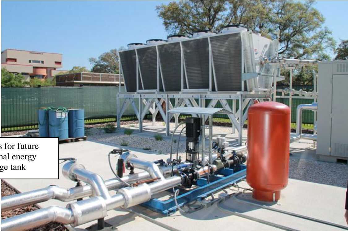
Fig. 5 Expansion tank and pump for the heat transfer fluid
