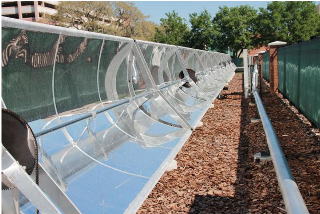
Fig. 4 A row of parabolic trough solar collectors
