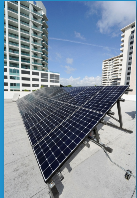
Solar panels on roof of Ft. Lauderdale Community Center
