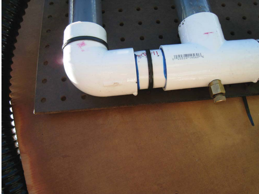
hydraulic fluid leak from improperly bonded PVC. The brass "pinch" plug on the right is used to calibrate the hydraulic fluid volumes.
