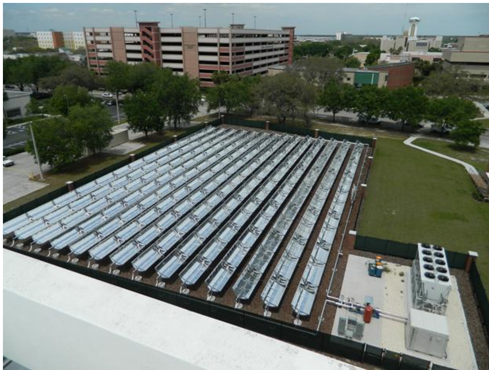
Fig. 1. Solar Field for 50 kW e power generation
