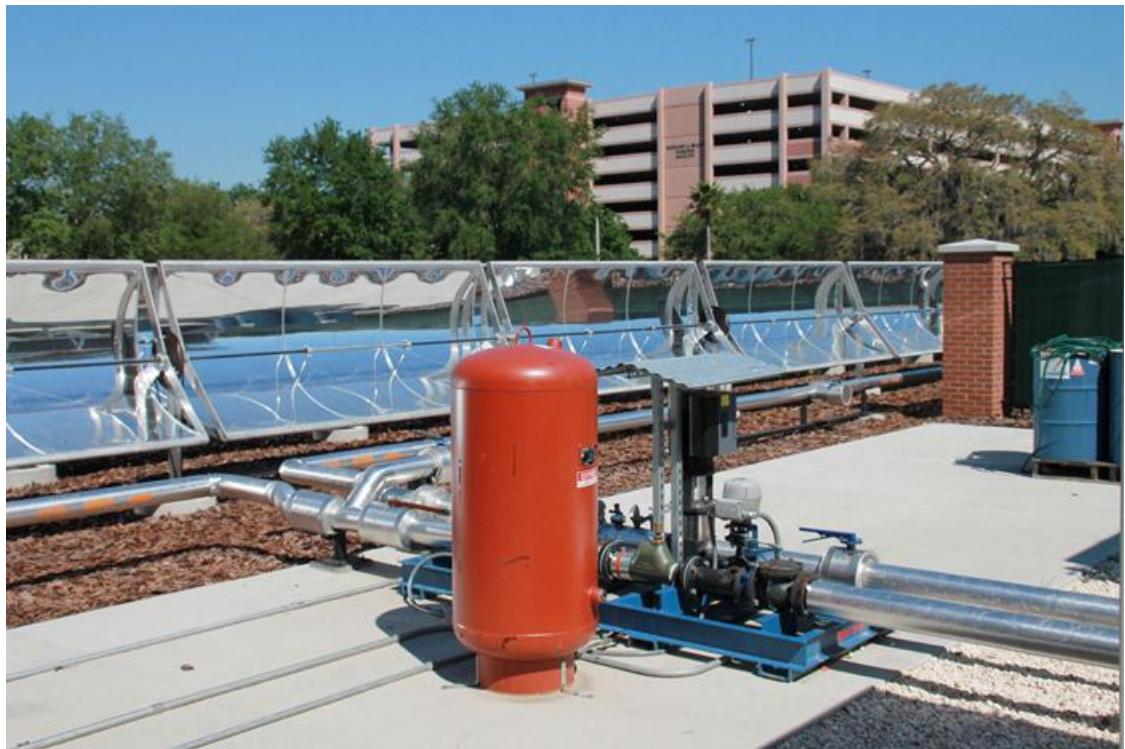
Fig. 6 Pump, piping and expansion tank for heat transfer fluid flow to and from the collector field
