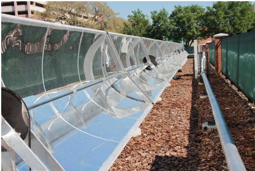
Fig. 4 A row of parabolic trough solar collectors
