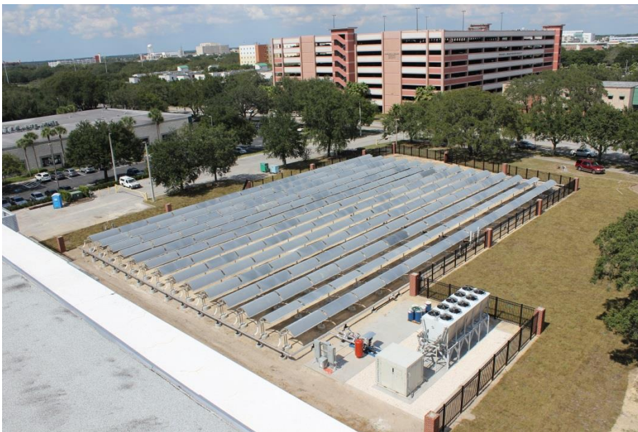
Figure 1. Solar Field and power block for the 50 kWe power generation system
