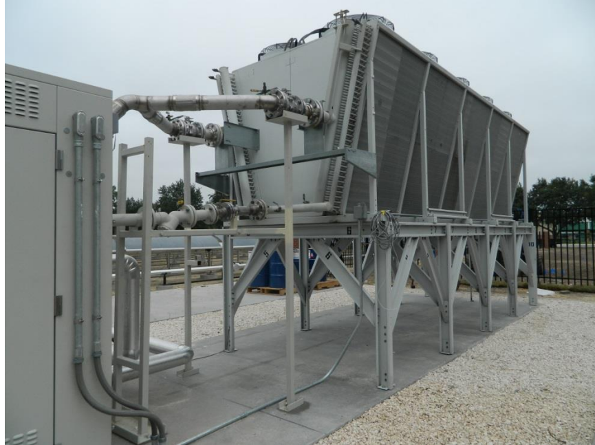
Figure 12. Electratherm power generator with air-cooled condenser.
