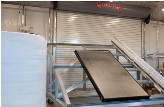
Figure 5. Solar Thermal Test Stand and Storage Tank (on left).
