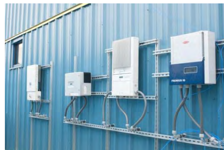
Figure 7: PV Inverter Testing
