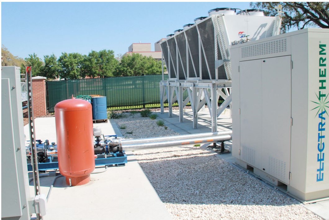
Figure 10 The Power block with the air-cooled condenser.
