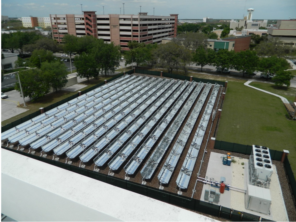
Figure 9. A view of the parabolic trough solar thermal power plant.
