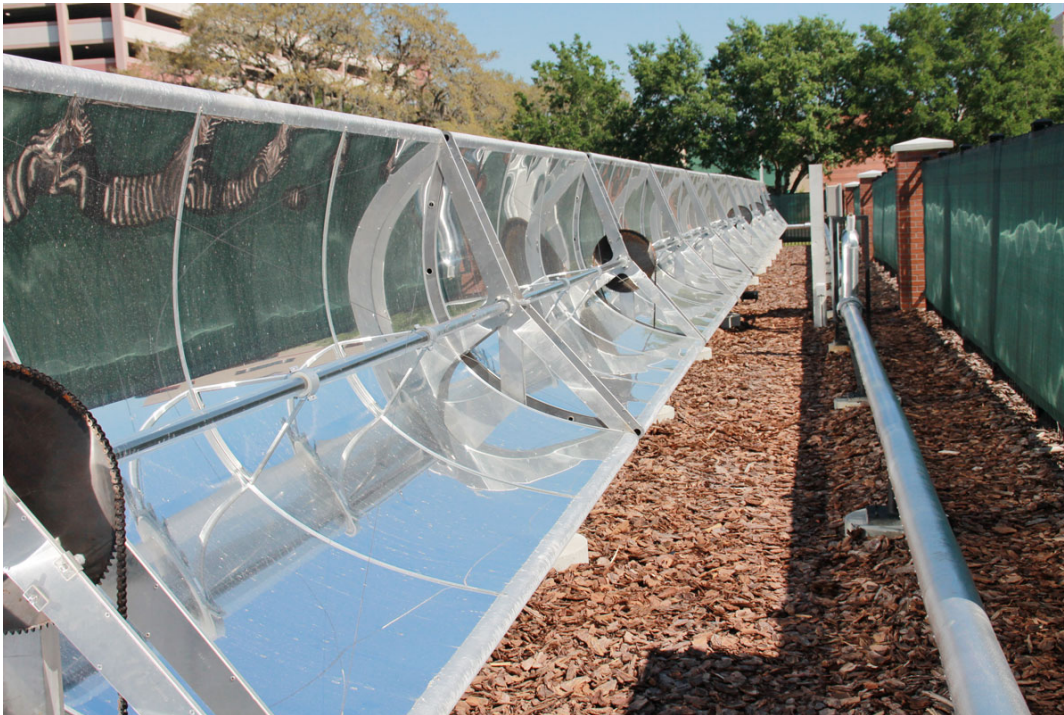
Figure 12 A row of parabolic trough solar collectors.
