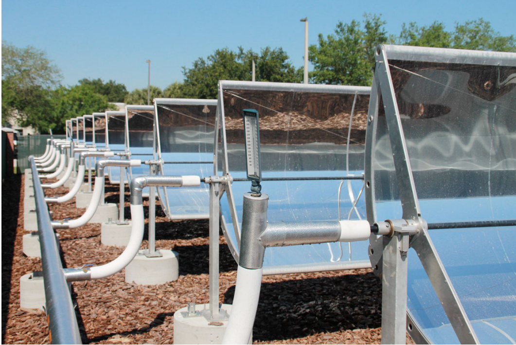
Figure 11 Solar collectors showing the header connections.
