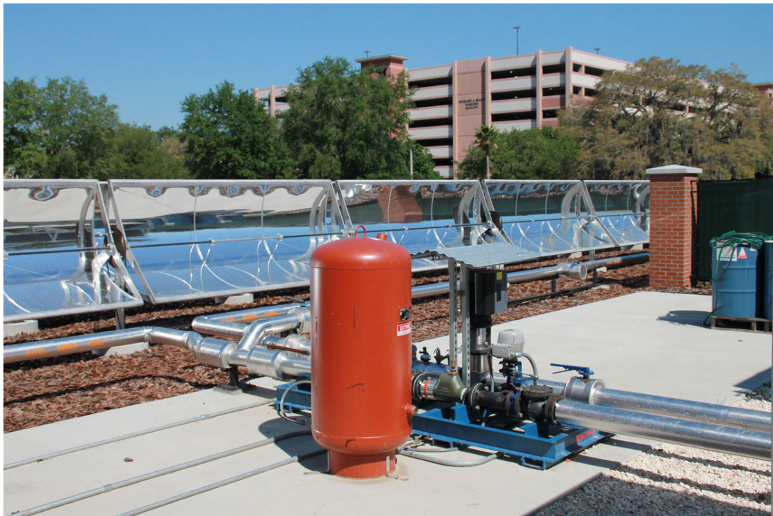
Figure 14 Pump, piping and expansion tank for the heat transfer fluid flow to and from the collector field.
